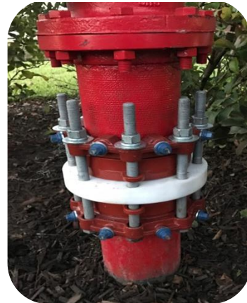
SMART VALVE™ 6" Installation
